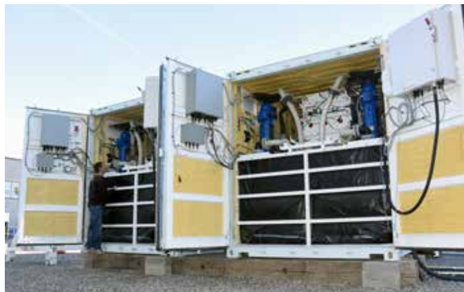
When filled with electrolyte solution, each of the flow batteries weighs approximately 25 tons. Together at full capacity they are capable of generating 128 kilowatts for 2.5 hours.
