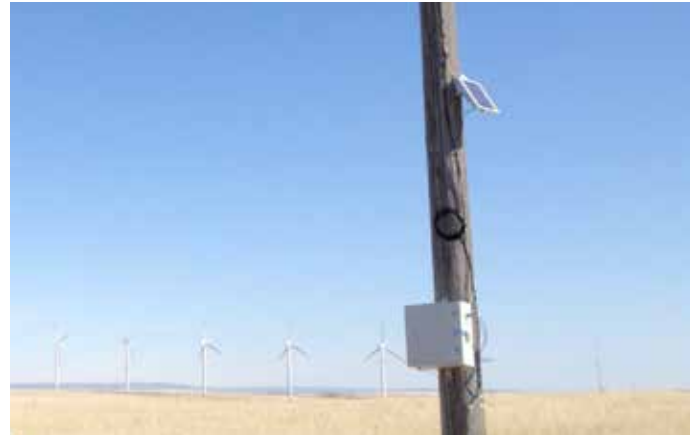
INL researchers and Idaho Power installed more than 40 weather stations along transmission lines in a windy part of southern Idaho’s interstate utility corridor.
