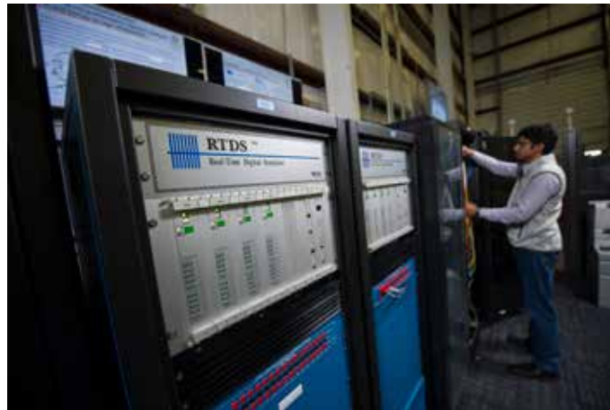
Thermal and electrical grid needs will be anticipated via a digital real-time simulator (DRTS).
