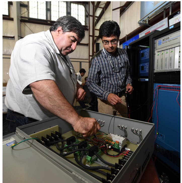
INL's Power & Energy Systems engineers use a Digital Real-Time Simulator to test hardware and controllers by emulating real-world grid events.
